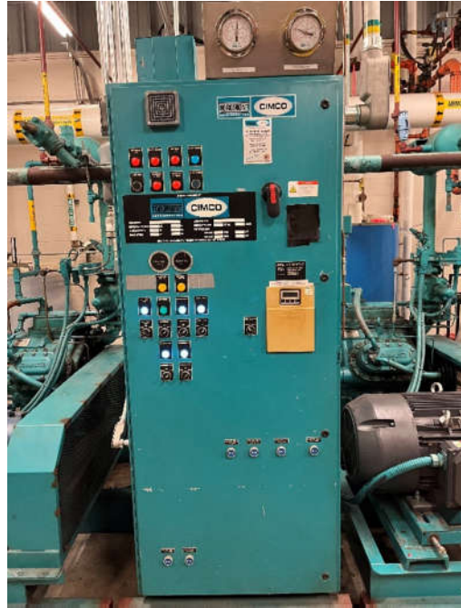
Figure 26: Cimco Refrigeration Plant Controller
