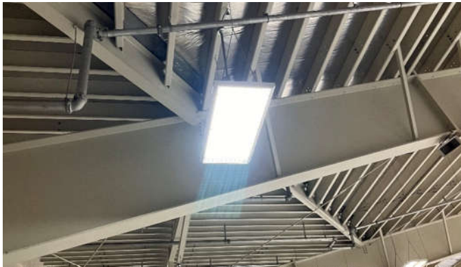
Figure 29: Typical Rink Area High Output Linear T5 Luminaires
