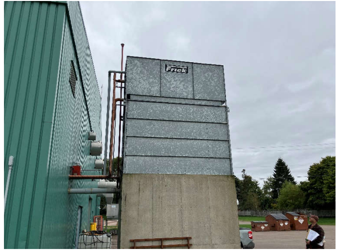
Figure 23: Ice Rink Refrigeration Plant Cooling Tower
