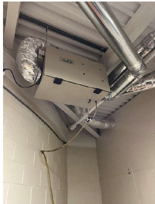
Figure 17: MTA Mounties Hockey Team Dressing Room Air Exchanger
