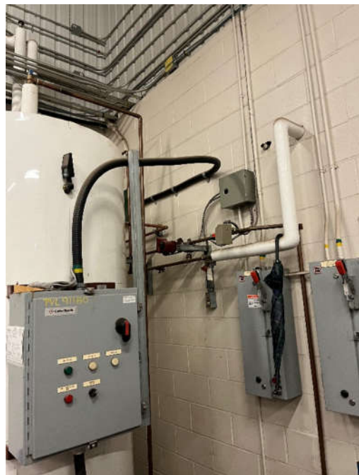
Figure 28: Rink Floodwater Tank System
