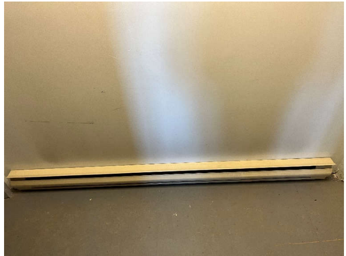
Figure 55: Typical Electric Baseboard Heater
