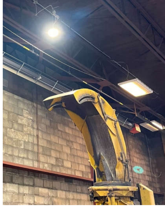
Figure 60: Typical LED High-Bay (Left) and High Output T5 (Right)
