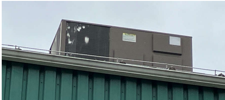
Figure 24: Typical Canteen and Fitness Area Rooftop Unit
