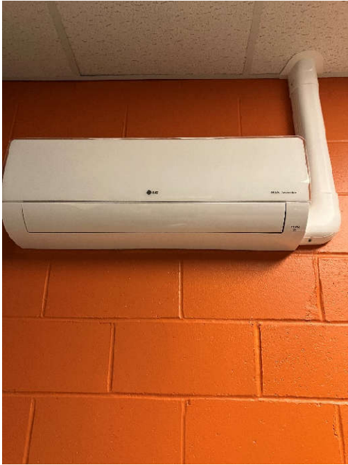
Figure 18: Mini-split Heat Pump in Reception Area
