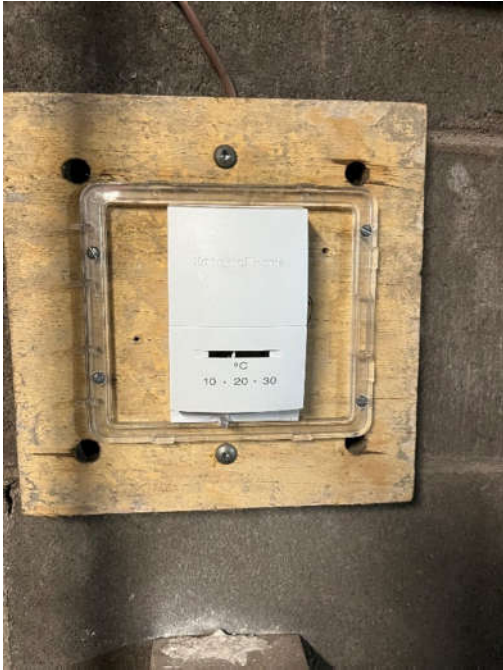
Figure 56: Typical Low Voltage Thermostat
