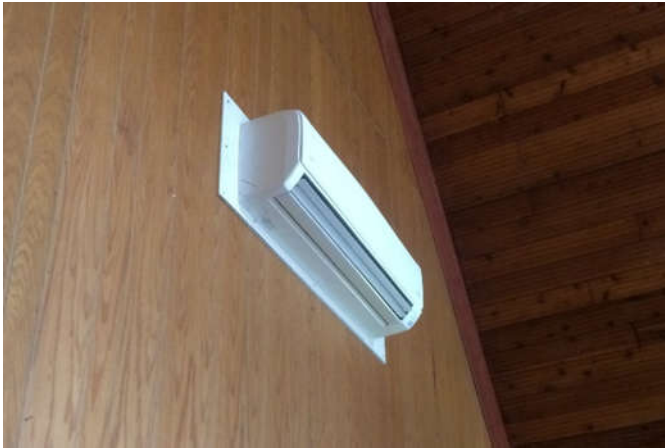
Figure 36: Typical Mini-split Heat Pump
