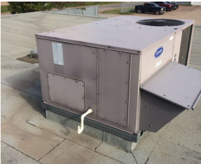
Figure 54: Carrier 5-Ton Packaged DX Rooftop Unit
