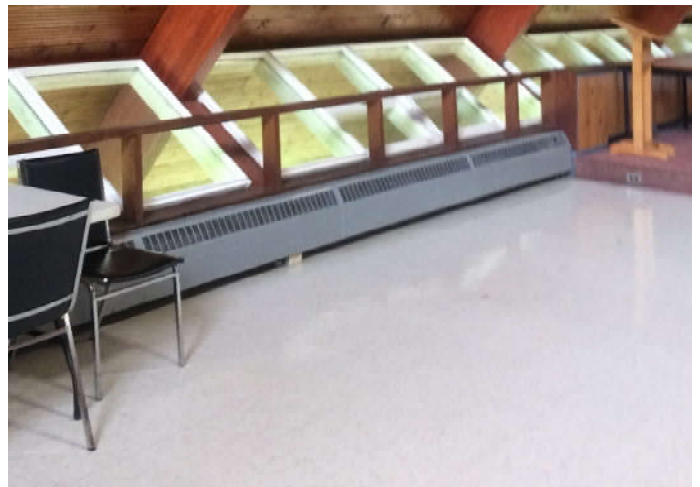
Figure 39: Typical Hot Water Radiators
