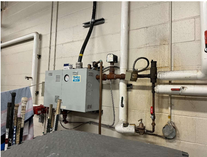
Figure 20: In-floor Heating Electric Boiler
