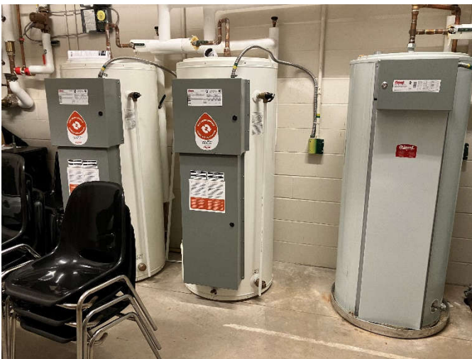
Figure 27: Domestic Hot Water Heaters (NB Power Rentals)
