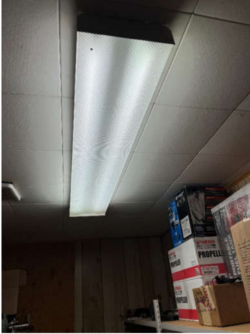
Figure 59: Typical Linear Fluorescent Luminaire
