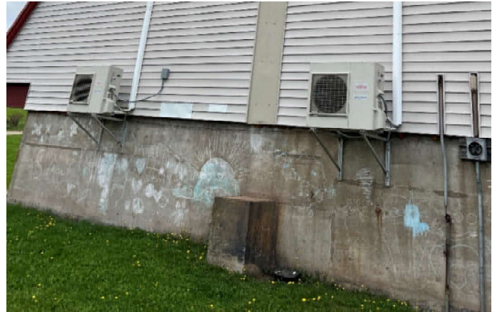
Figure 37: Typical Mini-split Heat Pump Condensers
