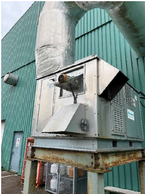
Figure 14: Ice Rink Area Dehumidifier (Not Operational)
