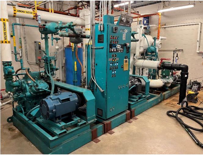
Figure 22: Ice Rink Refrigeration Plant
